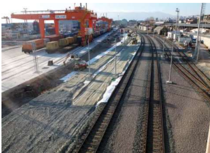
Figure 5: Gate/train operation area
